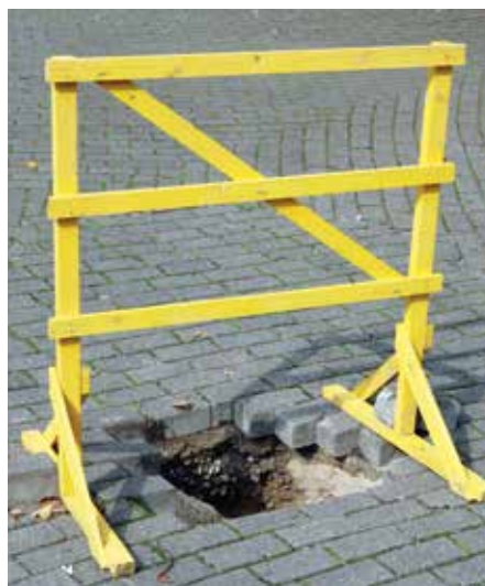
A ground hazard requiring a trench cover.
